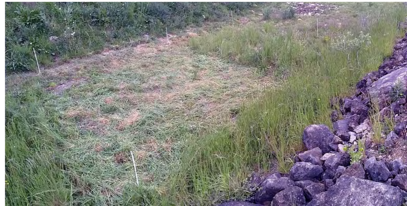
Figure 2: Establishment of one of the new demonstration plots in the quarry project.
